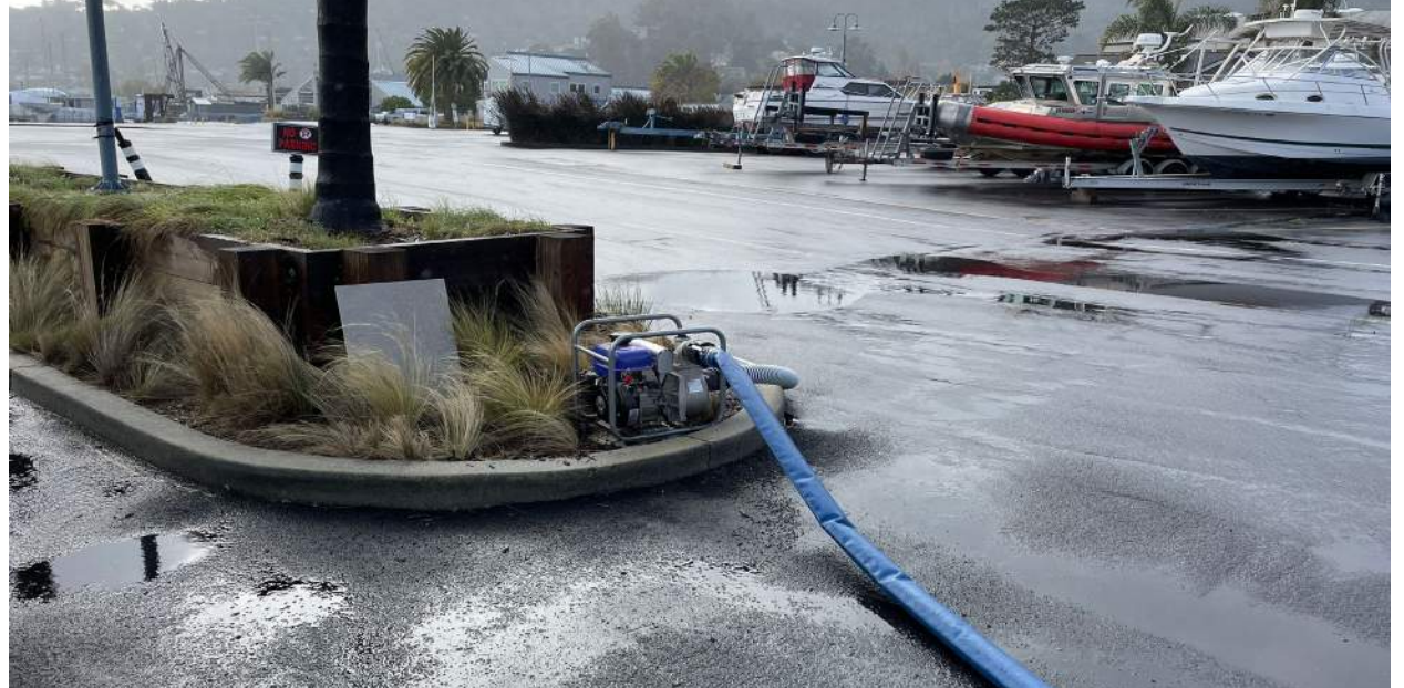
Pump Station at Work in a Parking Lot
